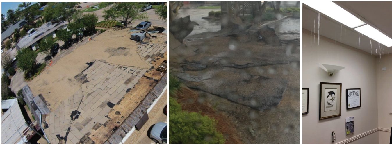
Figure 2. The destruction caused by the tornado to the roof (left), the parking lot (center), and the interior (right).
